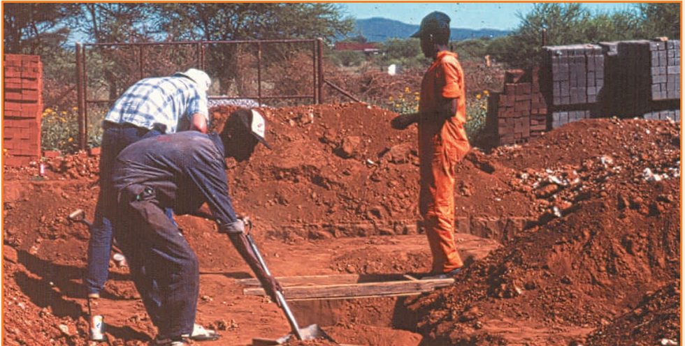
Figure 10 : Archaeologists rescuing cultural material exposed by foundation trenches of a house in Tlokwen, Southeastern Botswana.
